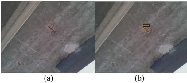
Fig. 6. Damage annotation in color images: (a) color image and (b) annotated image with damage.
