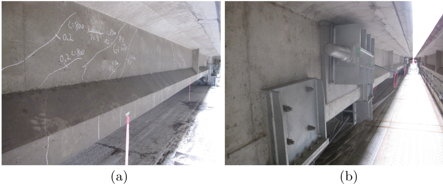
Fig. 6. a) Bending and diagonal cracks and b) External pre-stressing arrangement in a main girder
