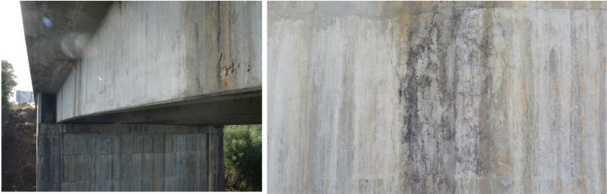
Fig. 3. Structural damage in the bridge.
