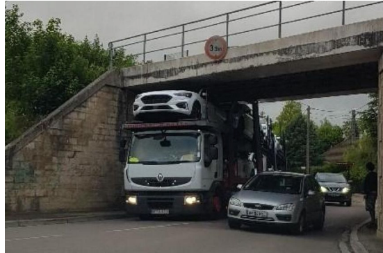
Fig. 1. The internet is full of examples of a truck hitting rail-bridges.
