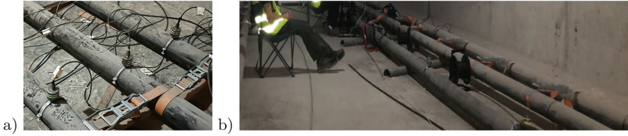
Fig. 3. Measurements of the dynamic response of the tendon during the tensioning process: a) accelerometers attached to the tendon using ad-hoc braces and b) Segment 5 supported on sheaths during the first stage.
