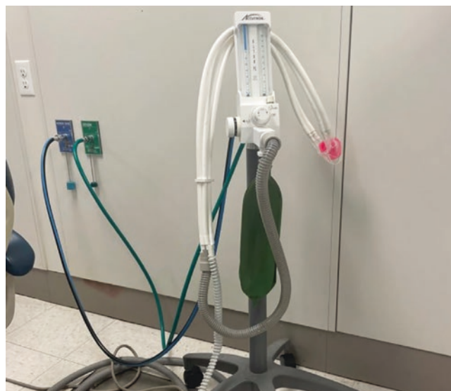
Fig. 29.2 An example of a nitrous oxide administration unit, including oxygen and separate nitrous oxide hosing
