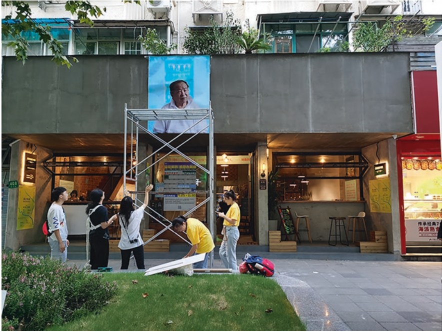
Fig. 5 Transformation of commercial space into exhibition space in Case C. Source: author, September 2021
