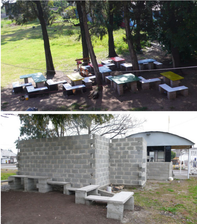
Fig. 26.13 Parts of the project built by the construction cooperative in Ciudad Roca Negra
