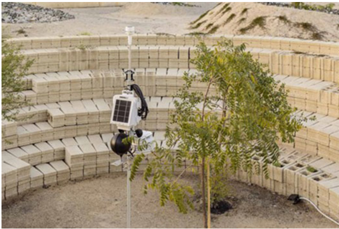
Fig. 11 Total station sensor installed at the center of the bowl
