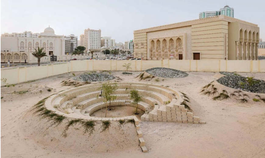
Fig. 12 Shot of the large central bowl during final phases of installation
