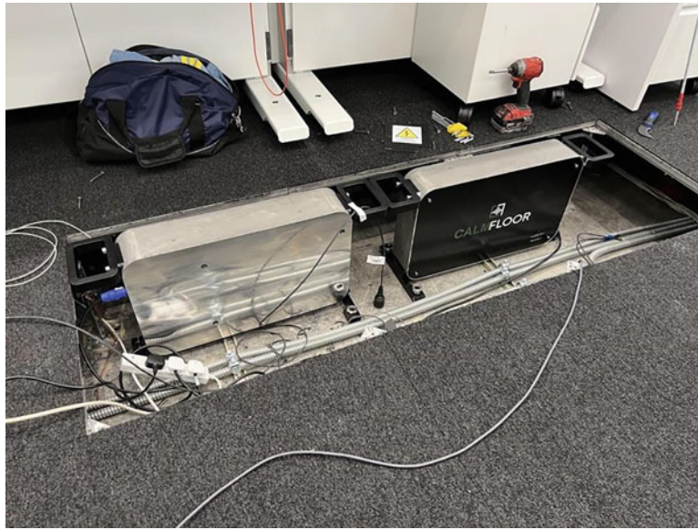
Fig. 25.5 CALM ® FLOOR AMD units and accelerometer used for FRF measurement at TP01
