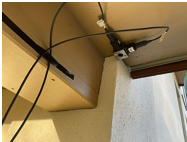
Fig. 1.3 An accelerometer positioned under a balcony at one of the corners of the building
