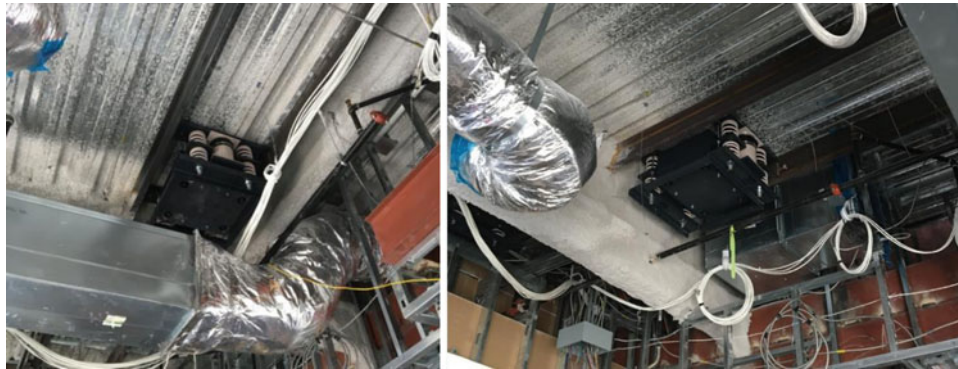
Fig. 33.14 Case 6 – Tuned mass dampers mounted to the underside of the floor structure
