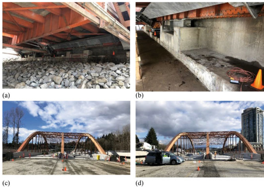
Fig. 7.11 Location of sensors on the bridge abutments and embankments: (a) sensors on abutment at east side (Setup 8); (b) sensors on abutment at west side (Setup 9); (c) sensors on embankment at east side (Setup 8); and (d) sensors on embankment at west side (Setup 9)
