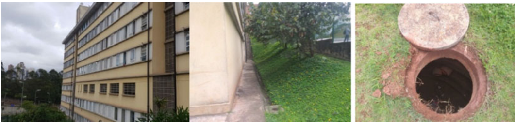
Fig. 2.7 Stormwater collection (Author, 2019)
