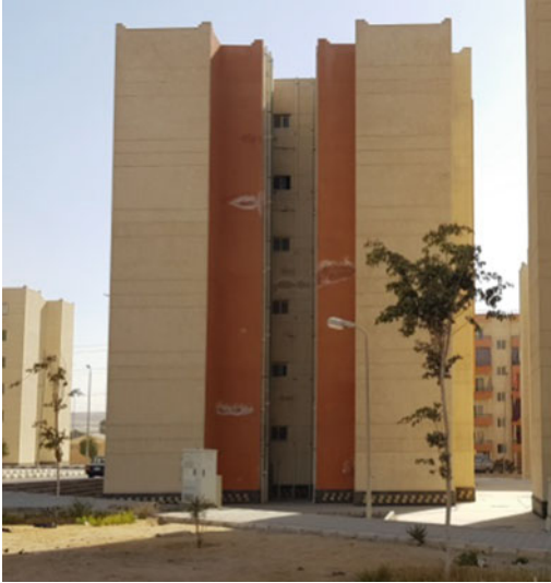
Fig. 2.3 Deteriorated facade (Author 2019)
