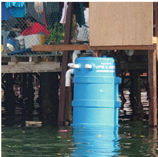
Fig. 4.6 One ISTP tank after installation below a toilet at Lok Urai water village. Source ACT Malaysia
