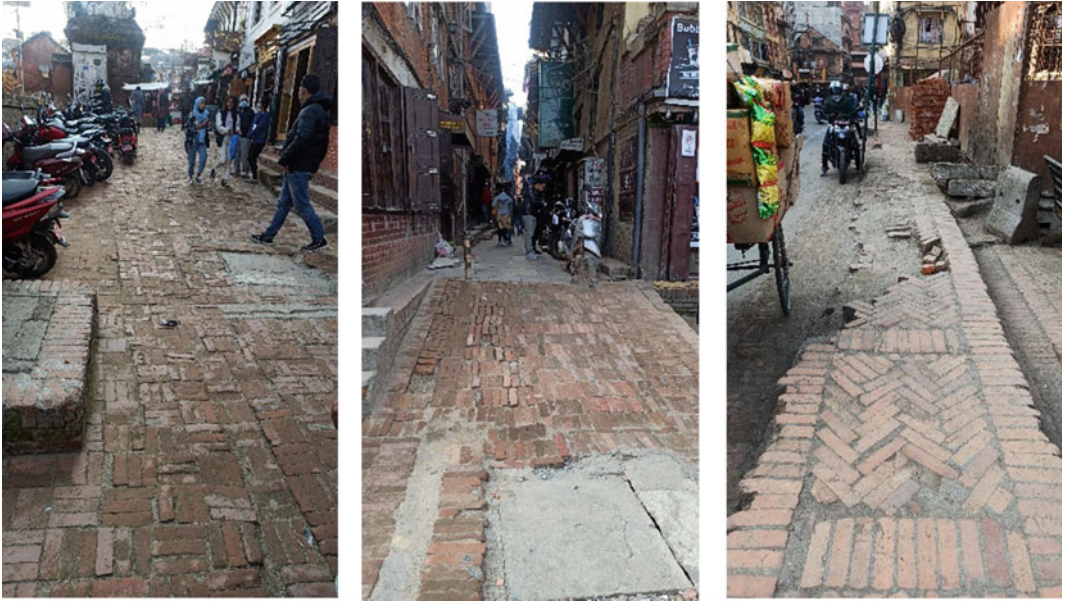
Fig. 18.10 Pathways in dire need of maintenance
