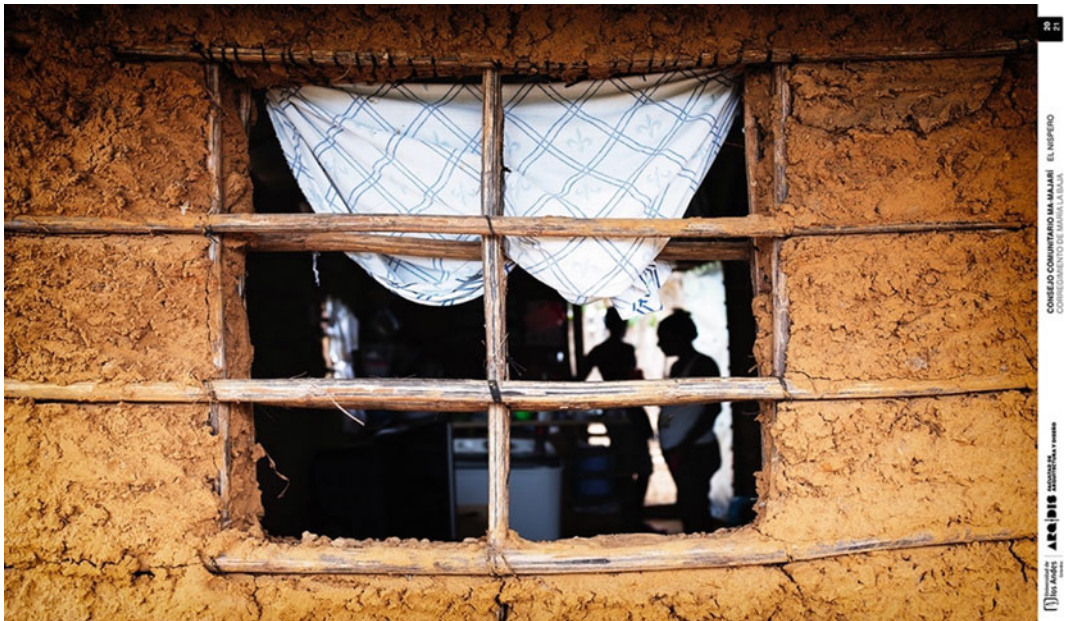
Fig. 6.49 “Bahareque” window in La Victoria neighborhood. Ma-Majari Community of El Nispero, Montes de María, Colombia 2021. @Daniel Huertas
