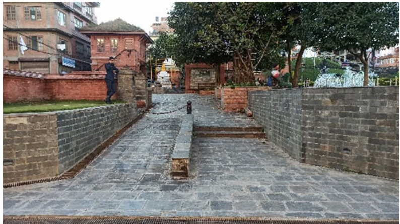
Fig. 18.27 Absence of handrails
