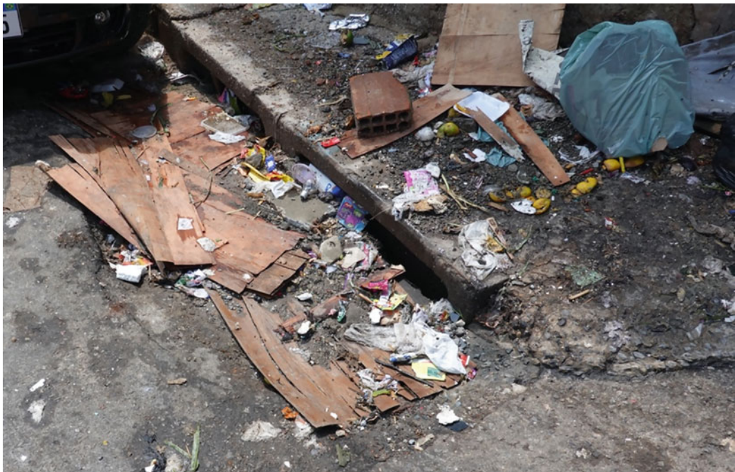
Fig. 42.2 Waste blocking out the drainage system
