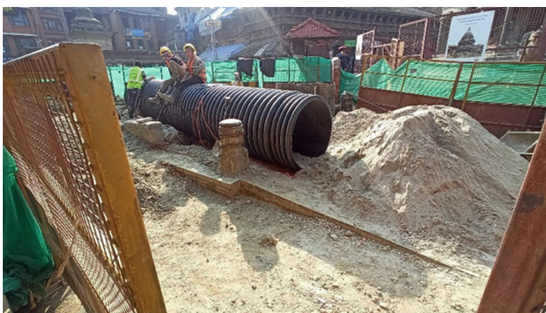
Fig. 18.6 The only ramp available at the entry of the square is frequently dug up for pipeline or roadwork
