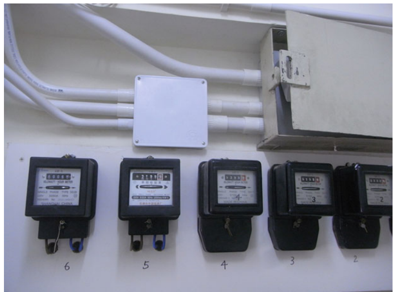
Fig. 41.2 Electric meters of a SDU, allowing different households to pay their own electricity costs (Courtesy Ka Wing Heung/Wikimedia Commons)
