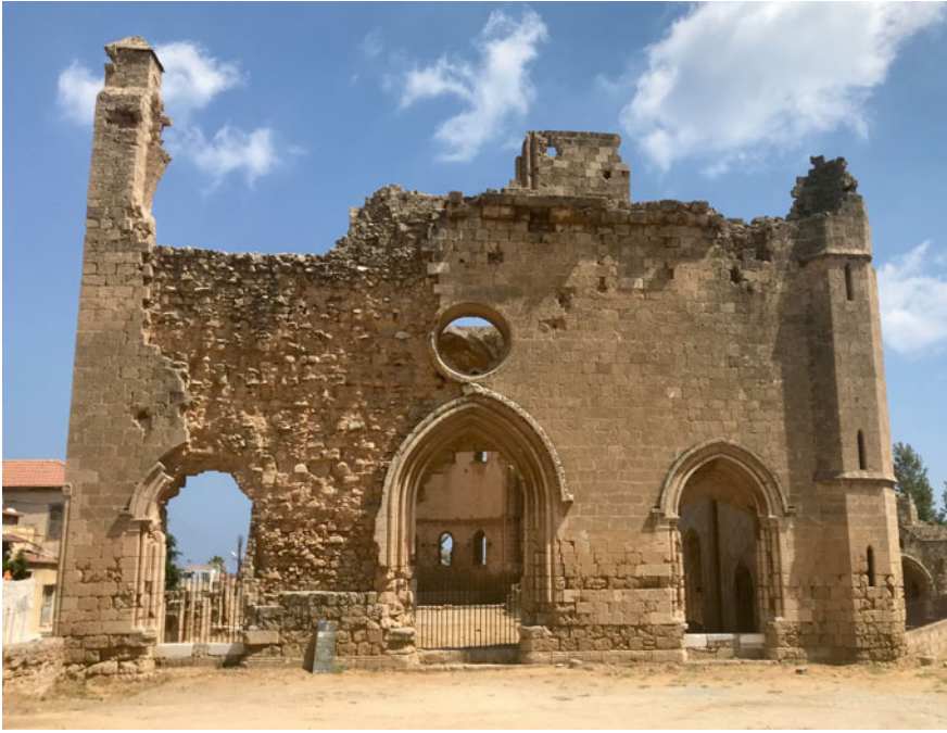
Fig. 1 Saint Gregory church in Famagusta found in advanced material decay and in need of structural emergency intervention for its consolidation and further preservation works. Photo by the Authors, 2021
