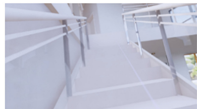
Slab is higher than the stairs
