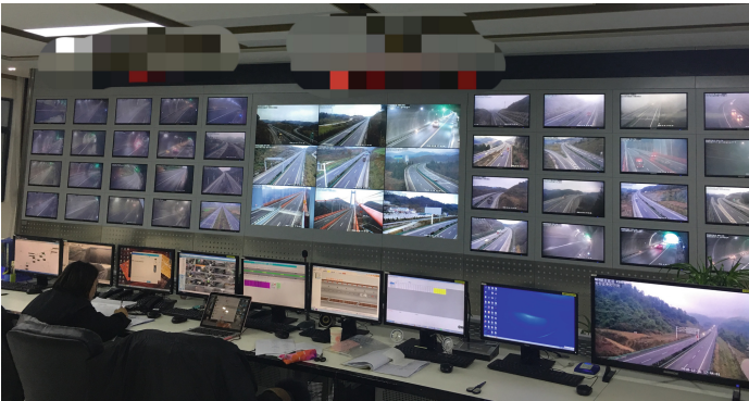
Fig. 1. A Chinese motorway control room investigated in this study.
