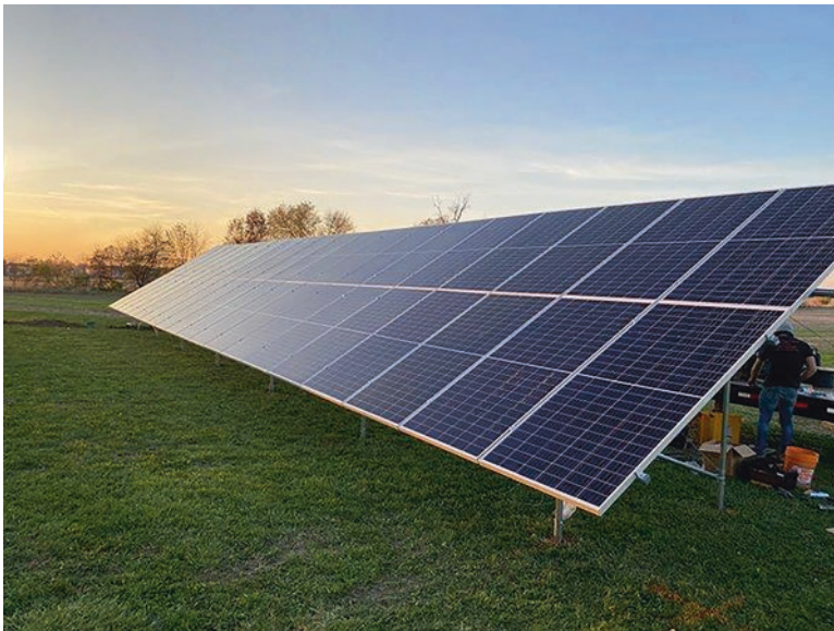
Fig. 9 Solar ground-mounted system
