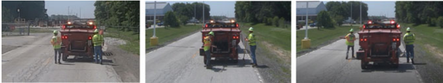
Fig. 2 Three activity classes identified for this study, crack sealing (left), transferring materials (middle), and walking (right)
