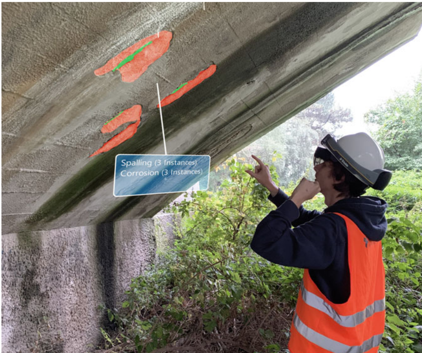
Fig. 1 Damage segmentation with the help of the HoloLens 2 on a bridge inspection mission.
