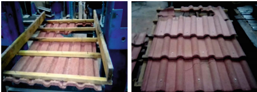
Fig. 8 Roofing tiles cracking and breaking in a row under the effect of applied uplift forces
