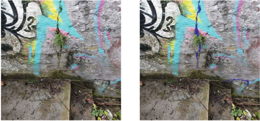
Fig. 9 Segmentation results with the FPN-Effb0 model. Blue color masks are crack predictions.
