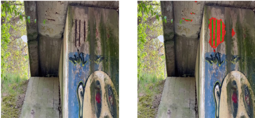
Fig. 7 Segmentation results with the FPN-Effb0 model. Red color masks are spalling predictions and green color masks are corrosion predictions.
