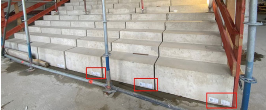
Fig. 3 Example of QR codes attached to prefabricated staircase on a construction site
