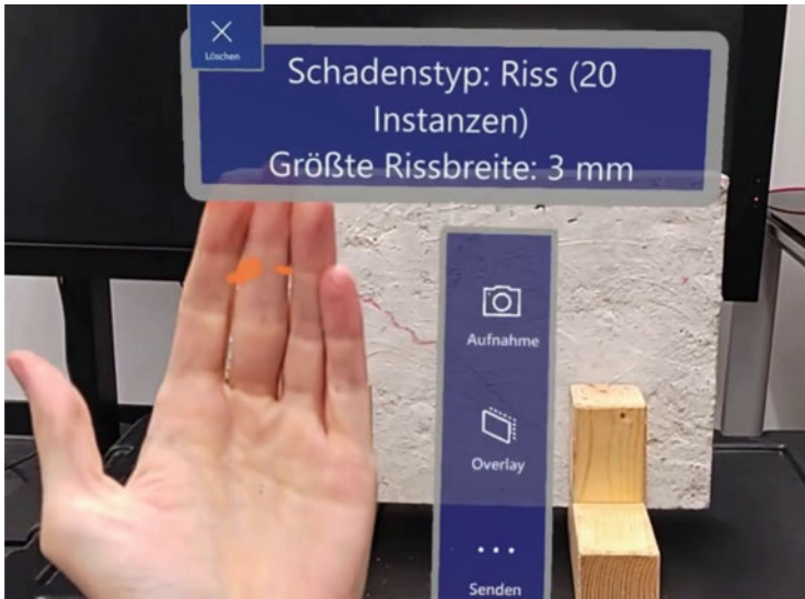
Fig. 6 Interface of the HoloLens 2 application. The functions for recording ('Aufnahme') and sending damage instances ('Senden') can be controlled through gestures and virtual interfaces. The crack in the concrete slab has been marked by the segmentation network in red.
