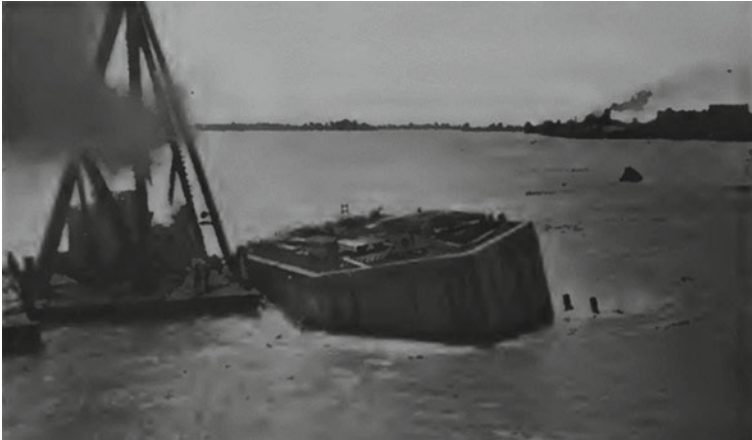
Fig. 6 Caisson 4 in distress. Source [2]
