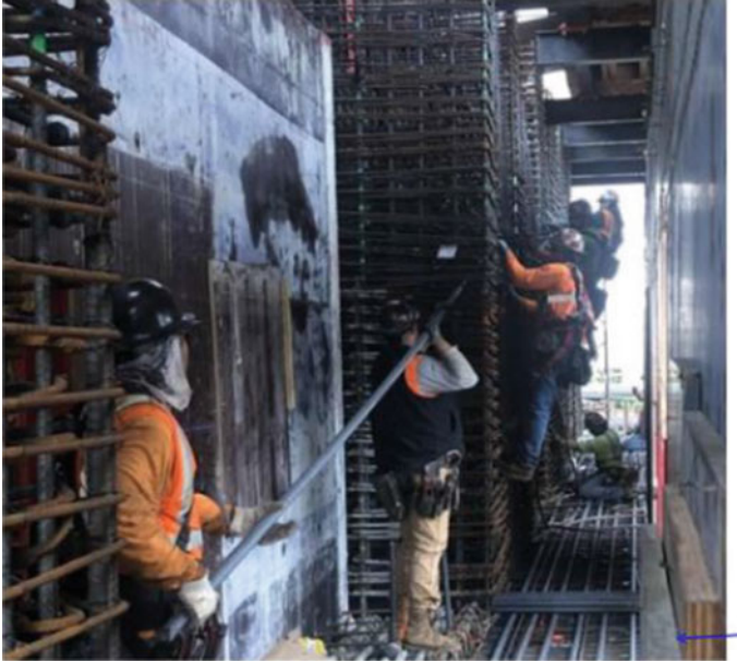
Fig. 2 Crew of five insert #11 (35 M) diagonal bars through wall boundary elements and into a diagonal coupling beam
