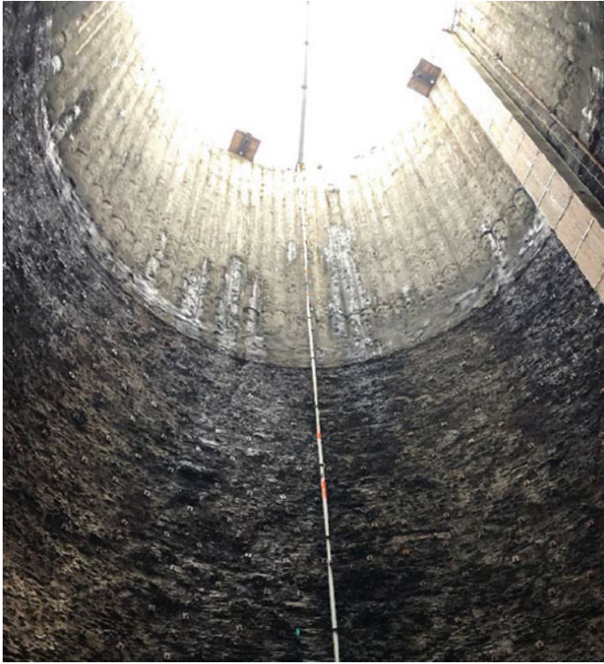
Fig. 3 Looking up from bottom of shaft at concrete caisson shoring and rock support
