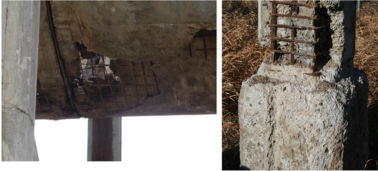
Fig. 13 Hole in the flume on the left and the base of a column showing loss of concrete on the right
