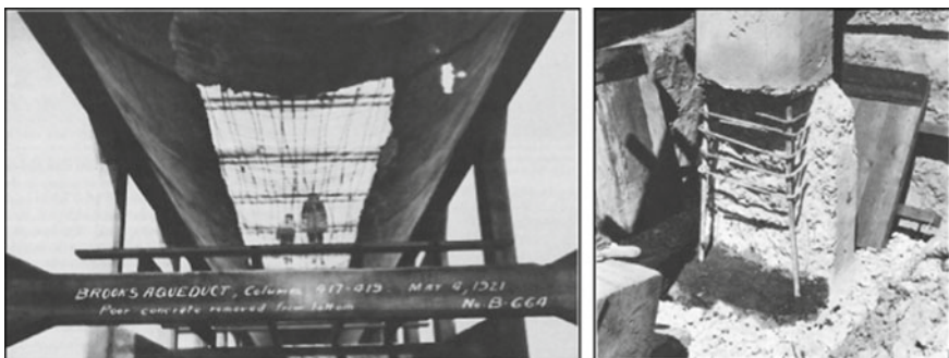
Fig. 12 Loss of concrete in the flume of Brooks Aqueduct (May 1921) and a footing (1927) as noted by Finch [2]
