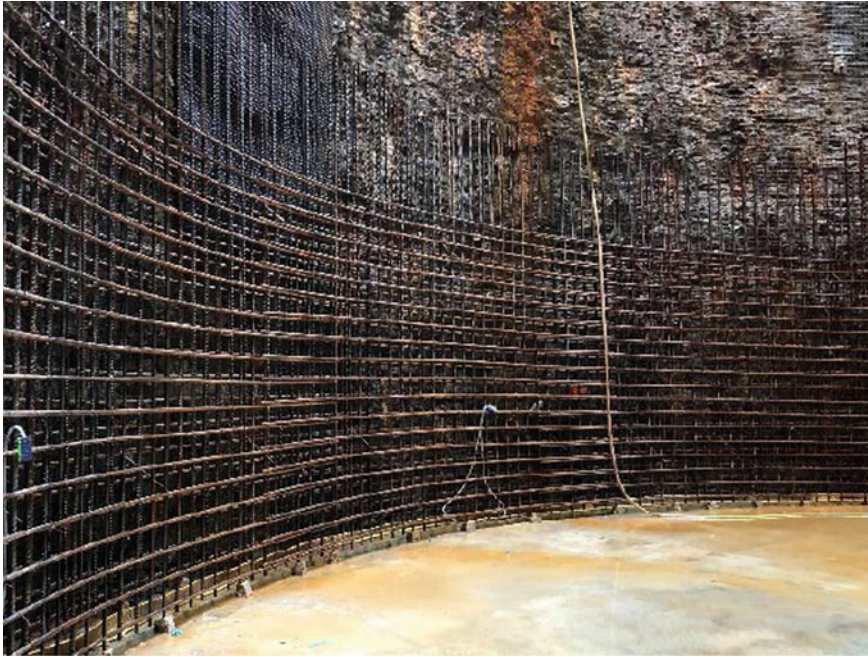
Fig. 9 View of typical rebar panel assembly for the first wall pour at the base of the shaft
