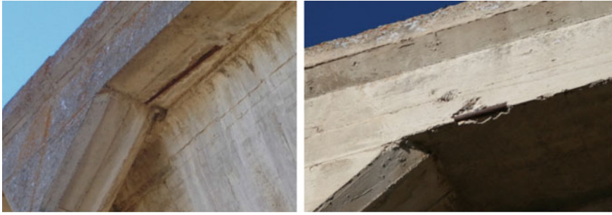
Fig. 5 Lack of proper cover for concrete—the reinforcing bars must have been touching the formwork in these parts of the Brooks Aqueduct
