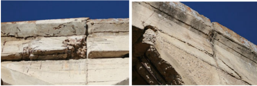
Fig. 10 Beams meeting at an expansion joint: the one on the left has been repaired at least once before, but there is a lack of stirrups holding the rusting longitudinal bar at the bottom of the beam: similarly in the beam on the right, the length and direction of the crack suggest that the stirrups and the angled longitudinal reinforcing bar were not placed as suggested in the schematic
