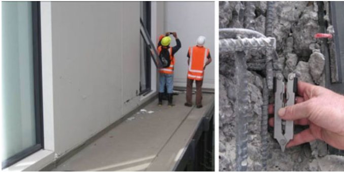
Fig. 2 Damage in RC wall in 2011 Christchurch earthquake [2] a crack at far end of the wall and b fractured reinforcing steel
