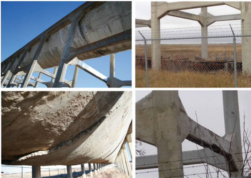
Fig. 14 Length of repaired flume is extensive as may be seen top left. Lots of forms were required with some shown top right. A geometric mismatch of the repair with the original flume is seen bottom left. Damage to the top and bottom of a crossbeam under an expansion joint is shown bottom right
