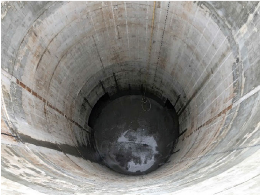
Fig. 10 View of completed shaft walls poured full circumference with no vertical construction joints
