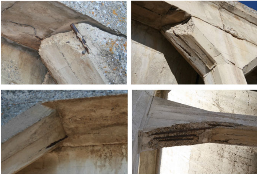
Fig. 6 Inconsistent placement of steel reinforcing bars, Brooks Aqueduct. Top left, a bar right at the front of a column head: top right, three bars all with virtually no cover in a column head: bottom left, a bar exposed at the rear of a column head: and bottom right, bars in a beam where it joins to a column—note the bars are not parallel
