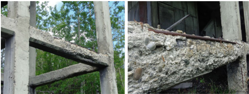
Fig. 7 Crossbeams in the frame supporting the Greenhill mine tippie structure—the minimal cover (about 10 mm) for the steel in the beams can easily be seen
