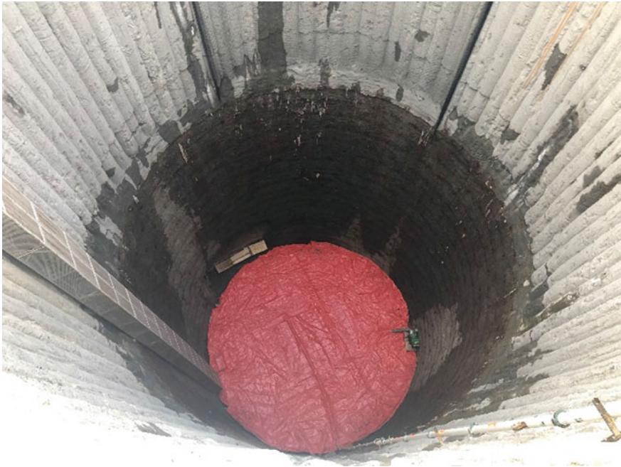
Fig. 7 Base slab curing underway with insulated tarps and portable heaters to control temperature differential of mass concrete element
