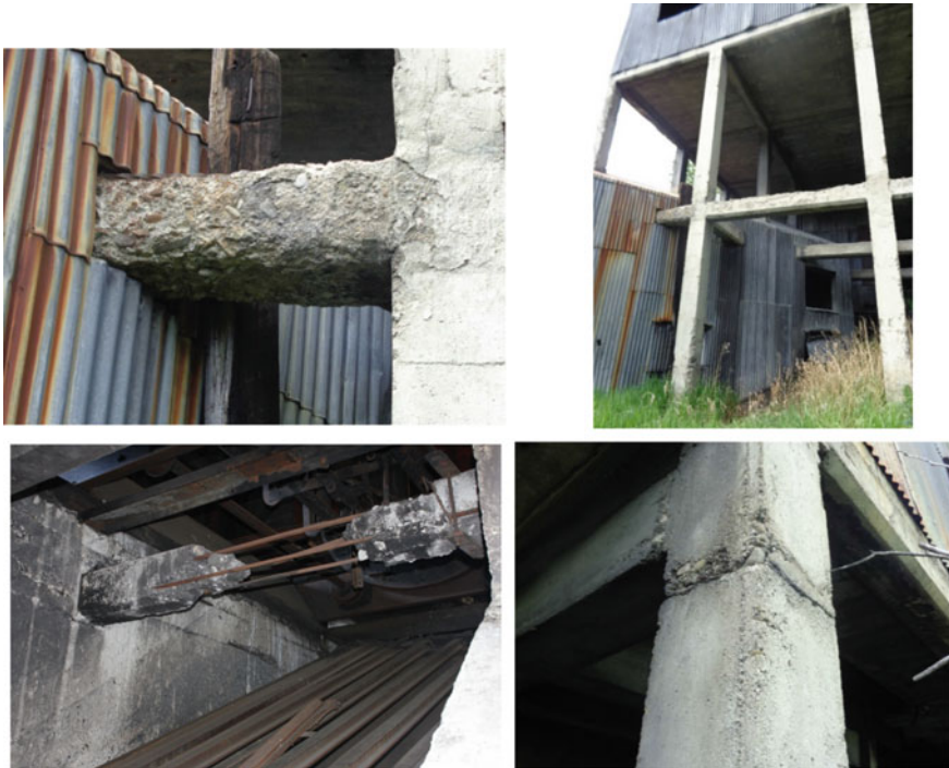
Fig. 15 Damage at the Greenhill mine tipple. Top left—flaking and spalling of a beam and the adjoining column. Damage to the top rather than the bottom of a beam (top right). Bottom left, complete loss of concrete in a beam under the slab where the coal was poured and a cold joint with minimal damage bottom right
