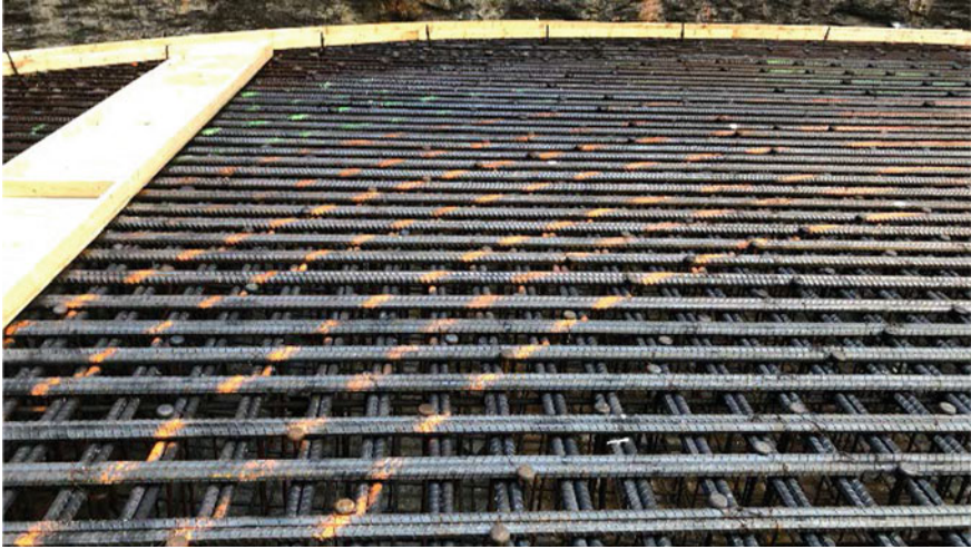
Fig. 6 Base slab top mat reinforcement consisting of 2–35 M bundled bars and radially placed headed shear reinforcement
