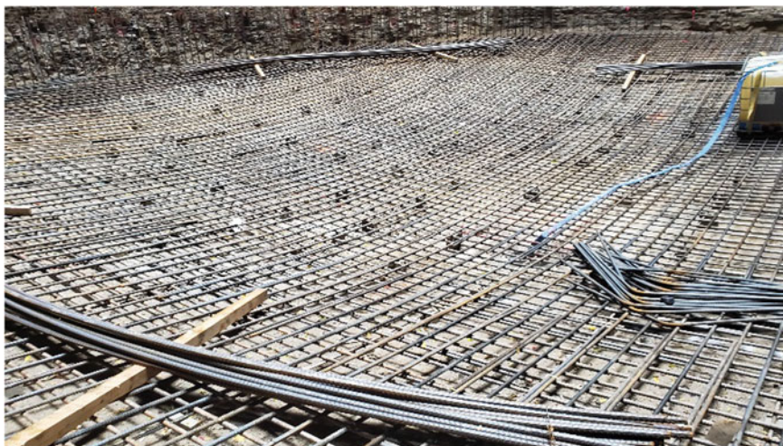
Fig. 5 Base slab bottom layer reinforcement, bars bent to the curvature of the hemispherical foundation
