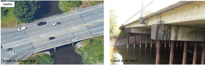
Fig. 1 Bird eye view of Kanaka Creek Bridge (left); substructure and steel pipe piles (right)
