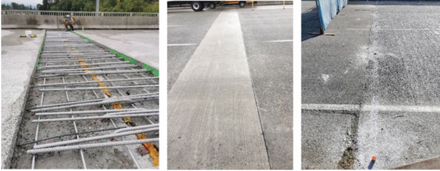
Fig. 9 Link slab rebar placement (left), finished link slab open to traffic (middle) and steel dowel drilling at abutment (right)
