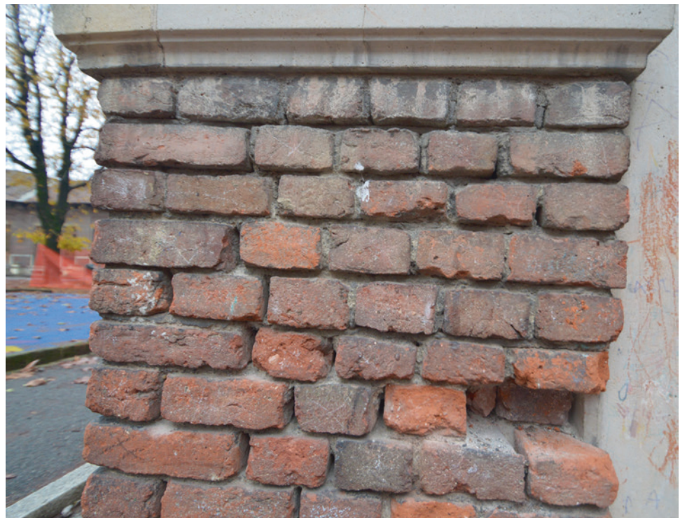
Fig. 10 Lack of mortar joints
