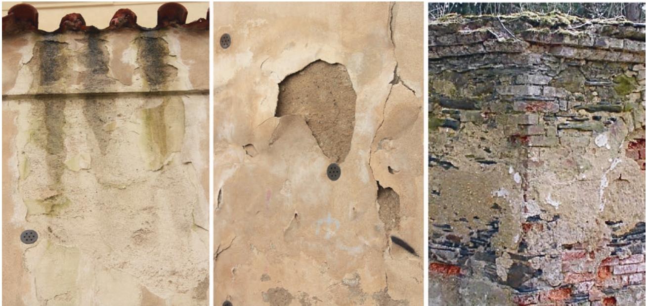
Fig. 4 Examples of damaged exterior plaster surfaces caused by increased humidity and related chemical, physical and microbiological degradation processes (photos by K. Kroftová, T. Čejka)
