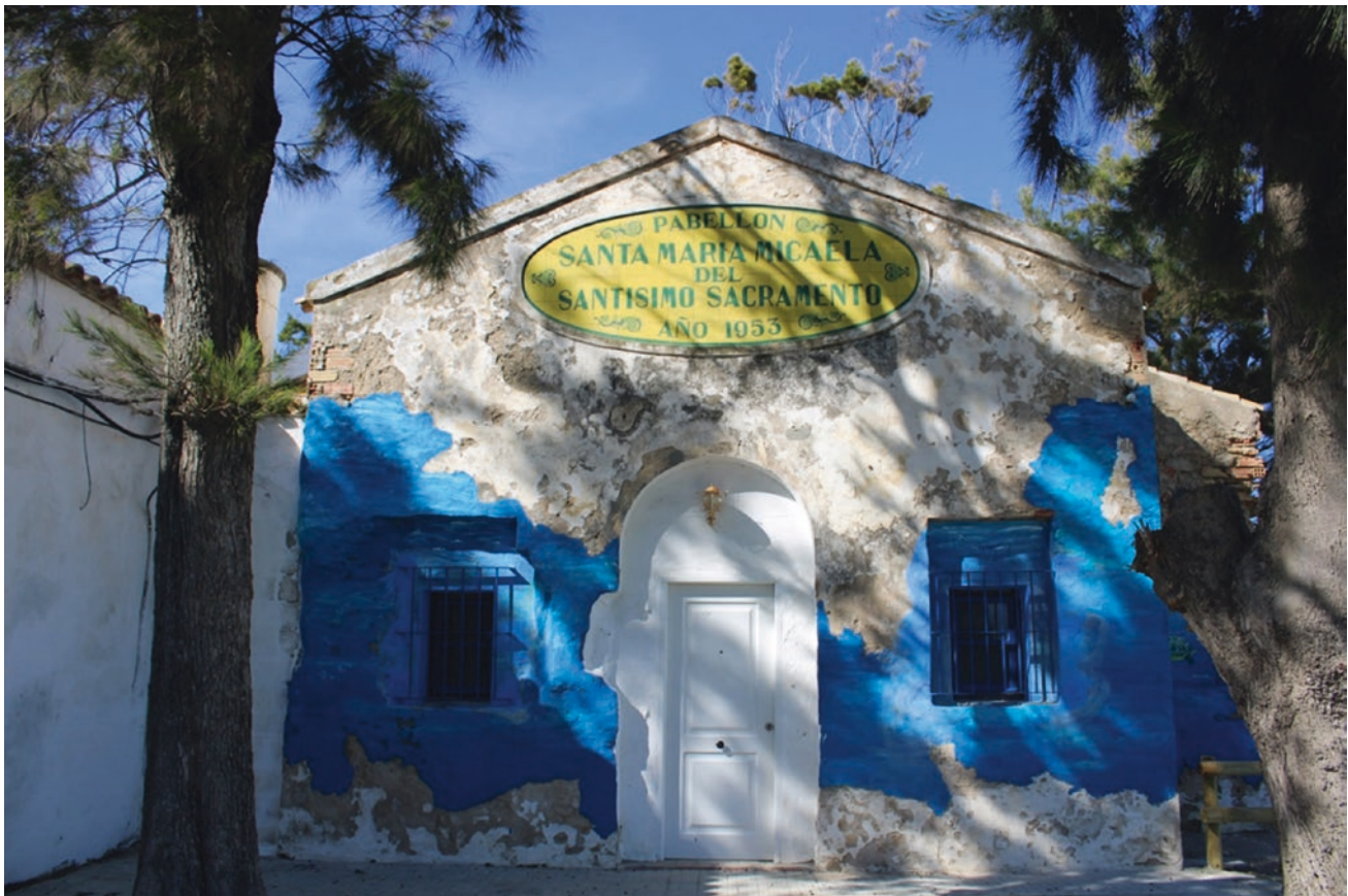
Fig. 4 State of the buildings in the town of Sancti Petri (Fernández Muñoz, 2022)
