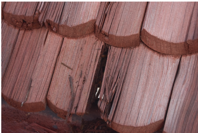
Fig. 5 Shingles damaged by rot. Photo Jennie Björklund
