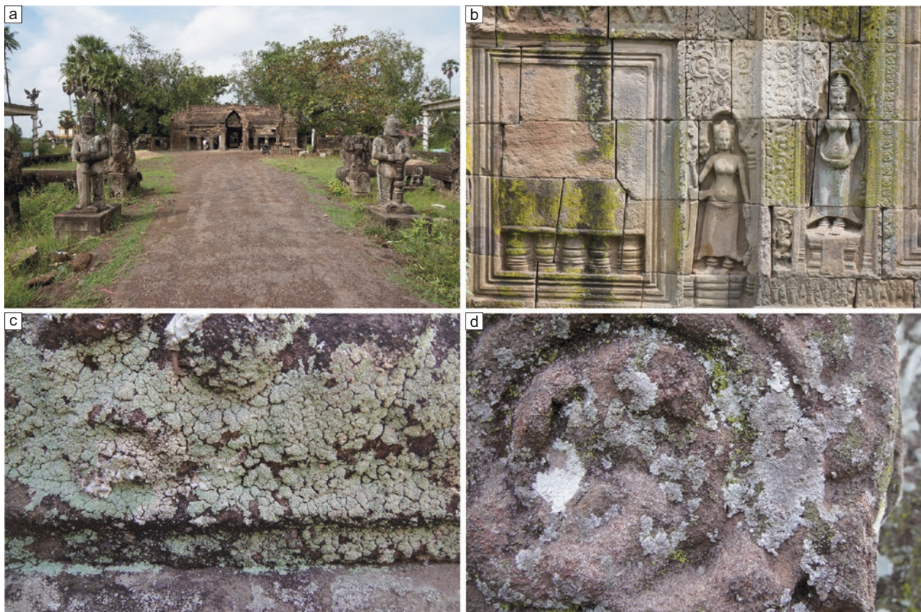
Fig. 1 Study object and biological weathering situation. a Main gate of the Nokorbachey Temple in the Angkor period. b Biological diversity on the sandstone gate. c, d Lichen on the stone block and lost part of bas-relief
