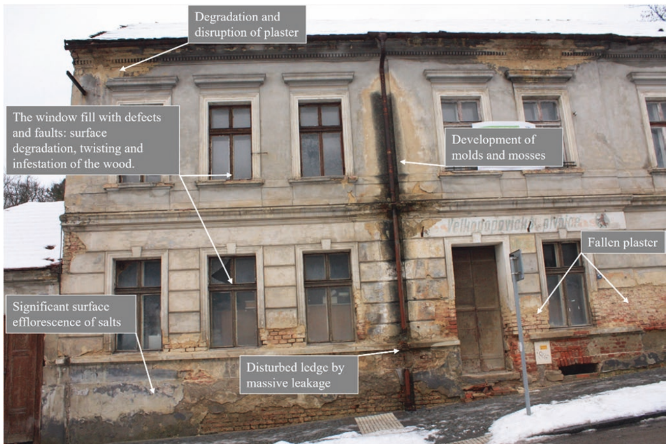
Fig. 2 The most common failures of structures from the second half of the nineteenth and the early twentieth centuries caused by degradation processes initiated in these cases by the combination of moisture, an incorrect design solution and neglected maintenance (photo by K. Kroftova)
