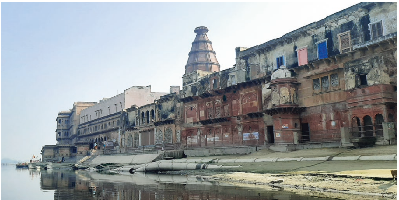
Fig. 7 Keshi Ghat of Vrindavan is in dilapidated condition, and there is no space left to perform any rituals. Source Author
