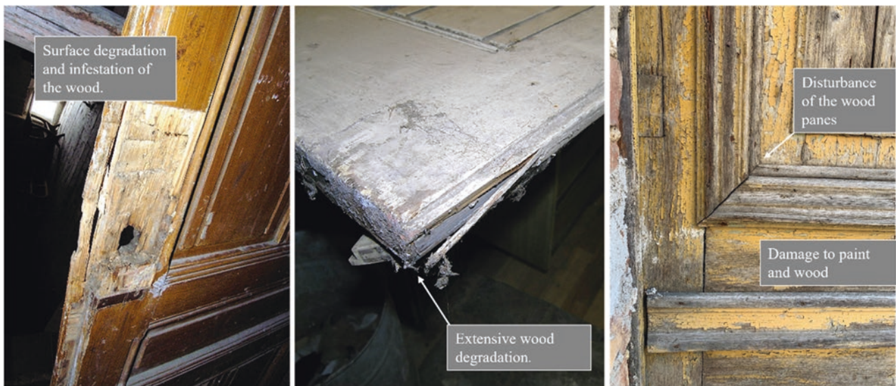
Fig. 7 Examples of the most common door wing failures—damage to the surface finishes and wood degradation
