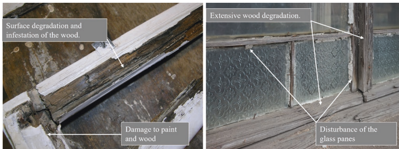
Fig. 6 Examples of the most common window failures—damage to the surface finishes, degradation of the window frame and damage to the sealant
