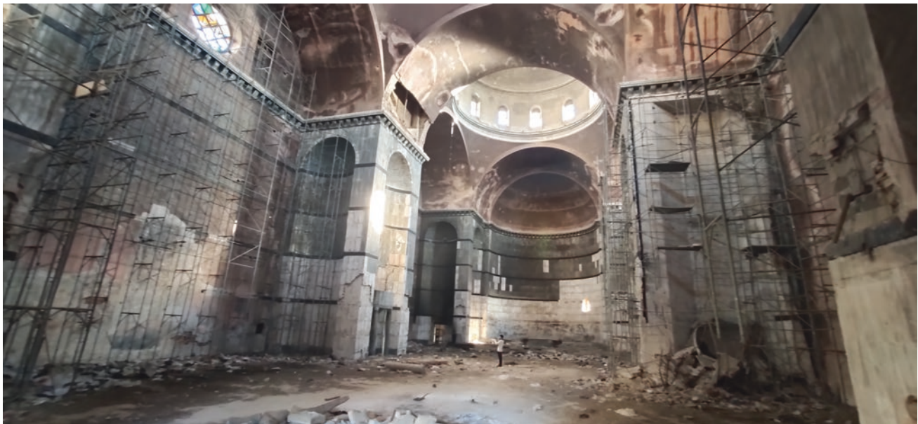
Fig. 5 Internal view of the presbytery of Benghazi Cathedral. Degradation phenomena caused by long neglect and manmade damage are evident (Photo by A. El-Rida, July 2021)
