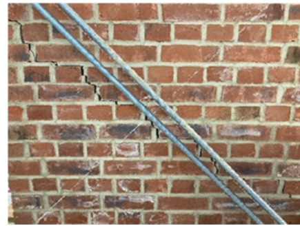
Fig. 16 Failure mode of a reinforced brick wall
