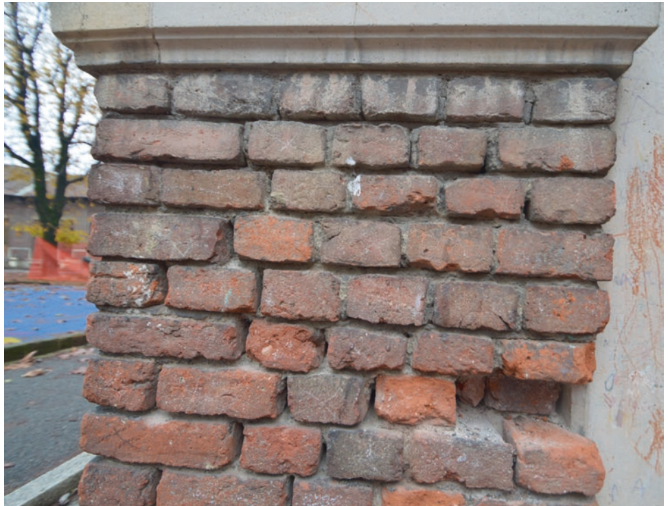
Fig. 10 Lack of mortar joints
