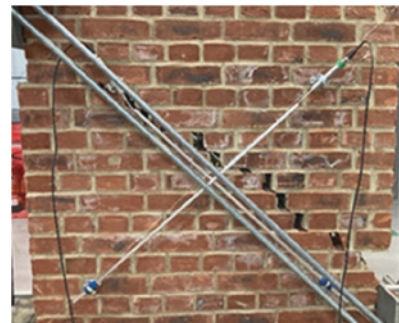
Fig. 13 Failure mode of an unreinforced brick wall
