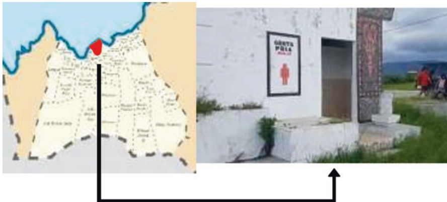
Fig. 10 State of public toilets on Lumban Bulbul Beach. (Source: Daritoba Project (April 2019))
