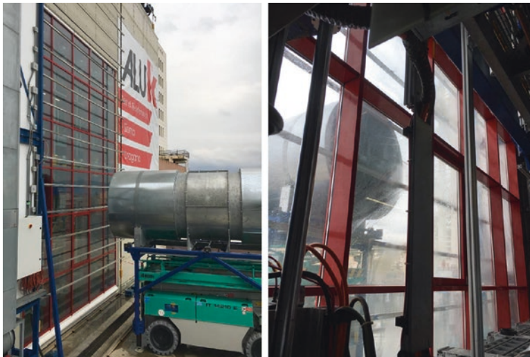
Fig. 5 Mock-Up tested for water-tightness under dynamic pressure (external and internal view). (Credit: TCLab)
