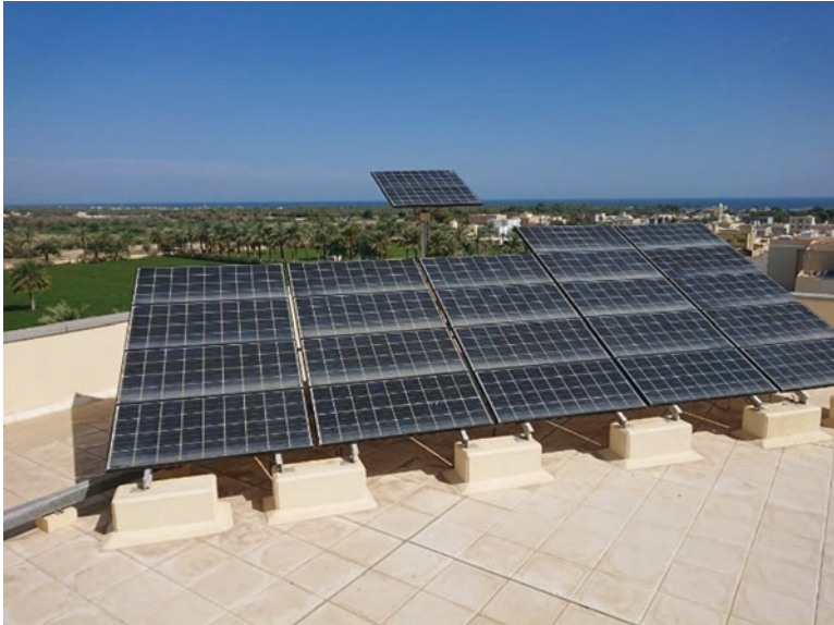
Fig. 2 Installed PV system
