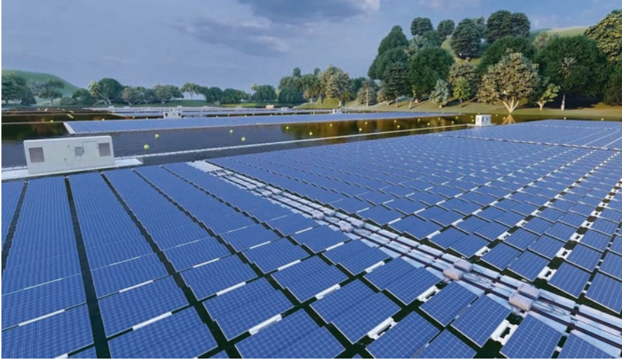
Fig. 15 145 MW CIRATA Floating PV Plant in Indonesia. The largest in Southeast Asia. It is supplying electricity to 50,000 homes and save 214,000 tons of carbon emission per year [12]
