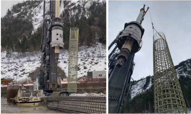
Fig. 7. GFRP cages in Gotthard Base Tunnel, Switzerland (Photos by Christoph Spitz, PohlCon GmbH, Germany).
