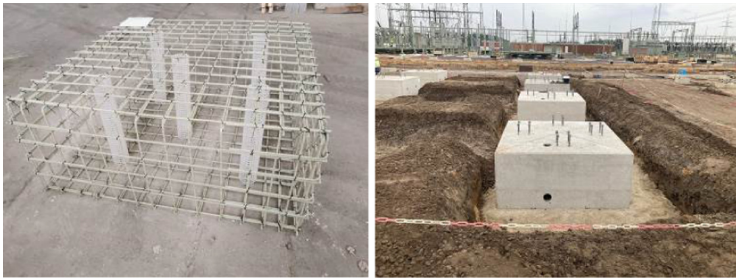
Fig. 4. Transformer foundation of electrical power plant in Germany (Photos by Christoph Spitz, PohlCon GmbH, Germany).
