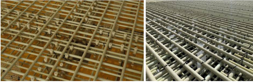
Fig. 3. a) GFRP shear reinforcement of Tokamak reactor slab, and b) GFRP bars in the slab of Zürich University Nuclear Medicine (Photos by Christoph Spitz, PohlCon GmbH, Germany).
