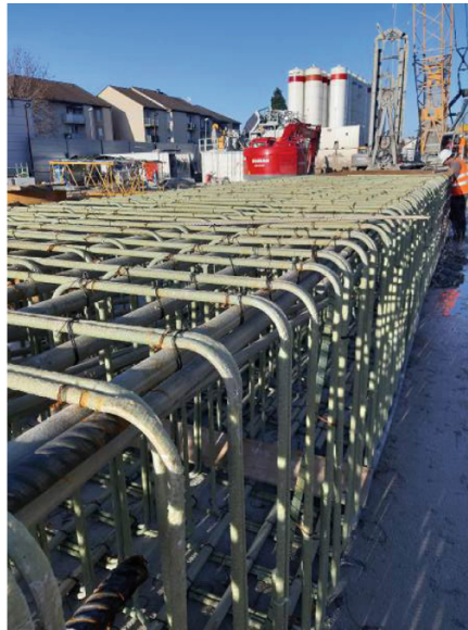
Fig. 6. GFRP in Grand Paris Express Tunnel (Photo by Christoph Spitz, PohlCon GmbH, Germany)
