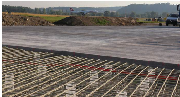
Fig. 5. GFRP in taxiways of Zürich airport (Photo by Christoph Spitz, PohlCon GmbH, Germany)
