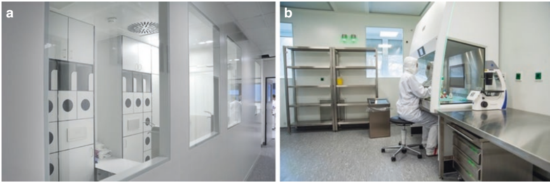
Fig. 2.7 Sterile room in the Klaus Faber Center for Cornea Diseases, incl. LIONS Eye Bank Saar-Lor-Lux, Trier/Westpfalz. (a) Decontamination corridor. The staff dresses in several steps through this corridor (cleanroom grades D and C) before arriving in the clean rooms grade
