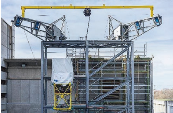
Fig. 8.8 Cable-driven parallel robot installed in the demo building. (Credit Alex Iturralde)
