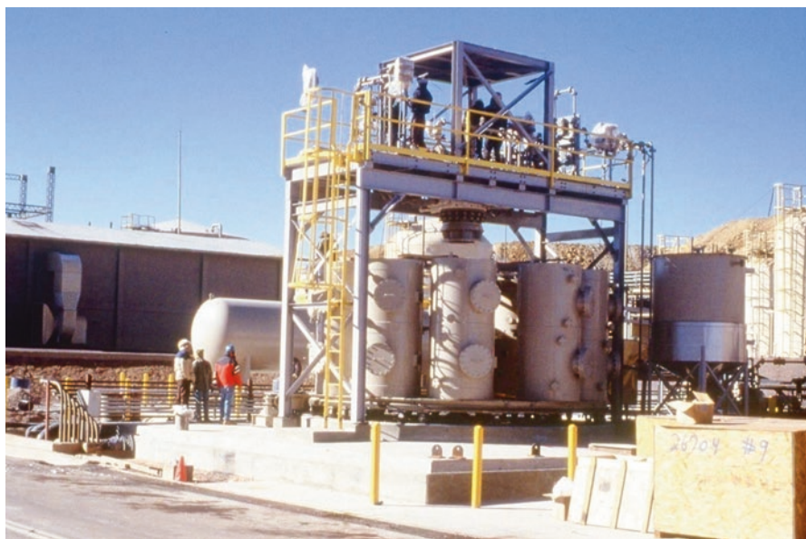
Fig. 7.3 CIX “carousel” type system installed at a copper mine in 1996 [19]
