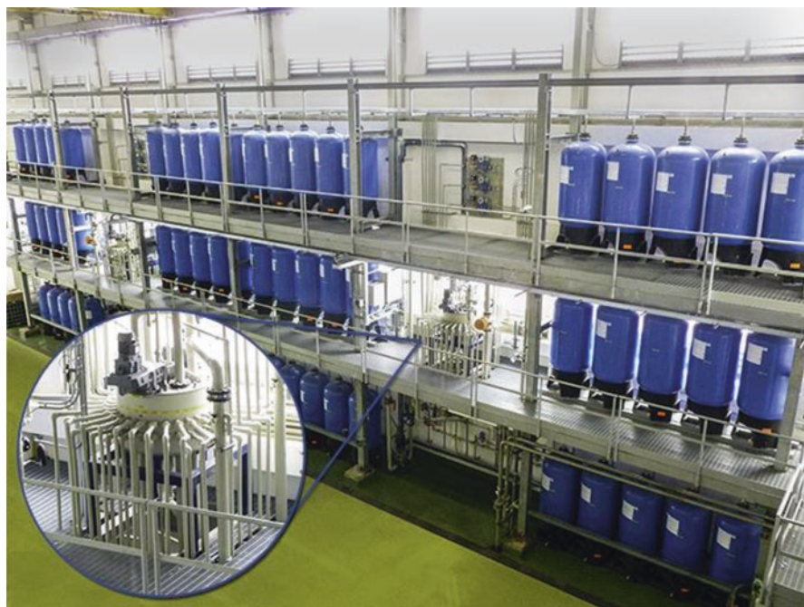
Fig. 7.6 CIX system alternative configuration over multiple levels. Two valves each controlling 30 columns. (Reproduced with permission PuriTech [23])
