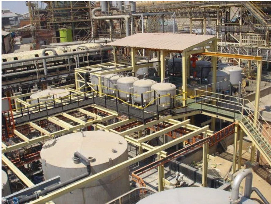
Fig. 7.5 CIX industrial-scale plant installation for metals purification. (Reproduced with permission PuriTech [23])
