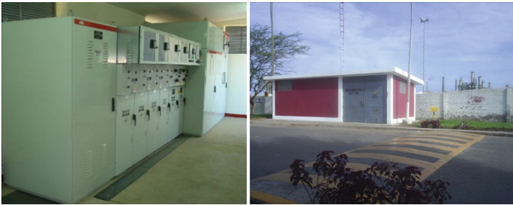
Fig. 4. Distribution of electric cubicles and substation photograph.
