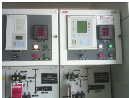
Fig. 7. Photo of Automatic Transfer System powered by ENOSA and Petroperú.
