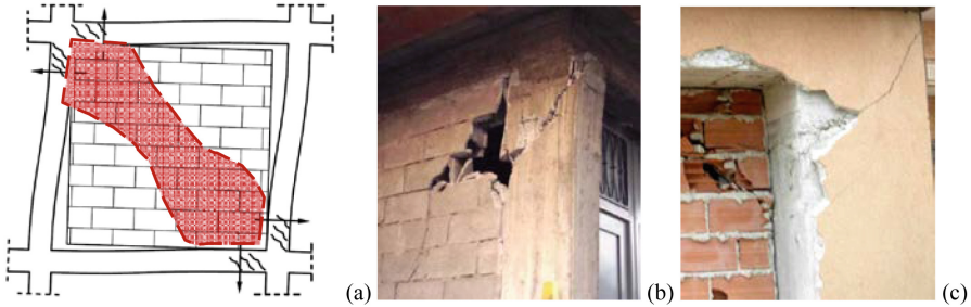
Fig. 1. (a) Local shear interaction of an infilled frame; (b) Shear failure at column ends; (c) Shear failure at column ends.
