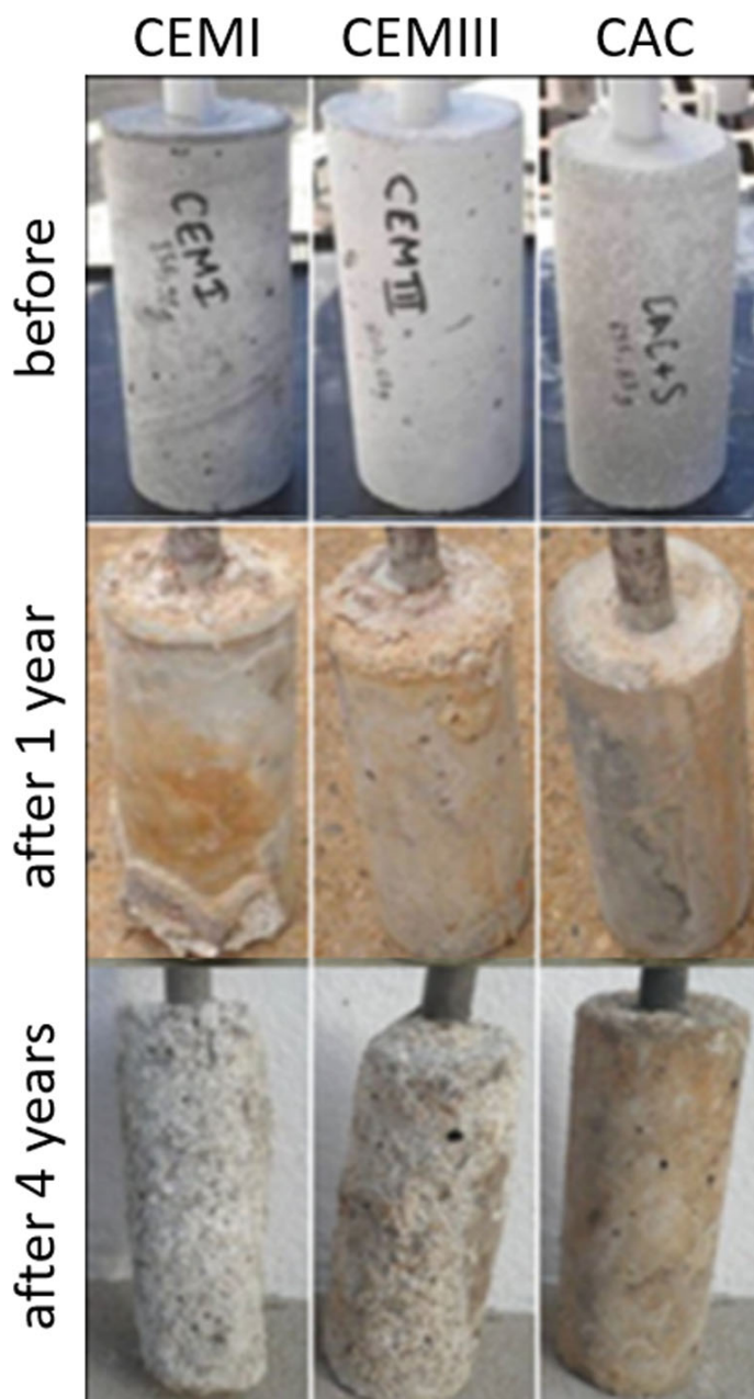
Fig. 1 Comparison of CEMI, CEMIII and CAC samples before, after 1 and 4 years of exposure in a sewer system. Adapted from Herisson et al. [39] with permission from Elsevier
