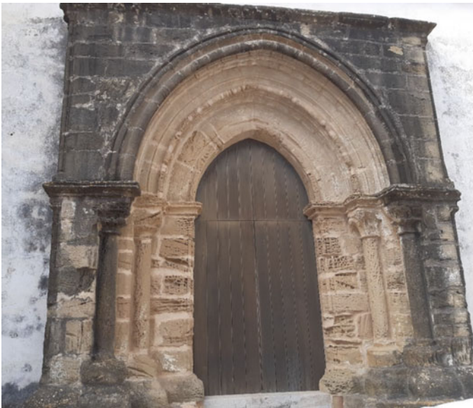
Fig. 1 Portal of St. Leonard's South façade showing alveolization patterns
