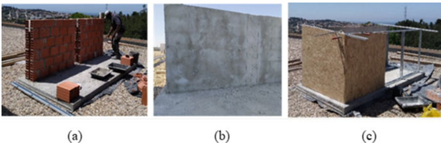
Fig. 5 Construction of the test cell: a cavity wall being constructed; b the wall after plastering; c the wall after thermal insulation
