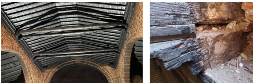
Fig. 1 General and detail images of the state after the fire of the church of San Martín (2020). Image source OCR-Extremadura
