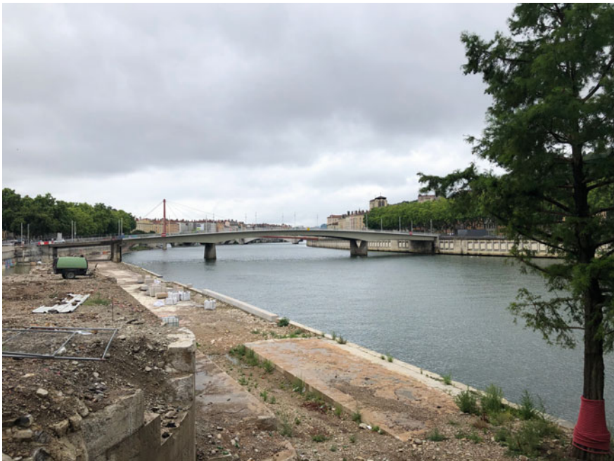
Fig. 9.2 Creation of a river garden on the Terrasses Presqu'île in progress with demolition of the old mineral quays (Source Seigneuret 2022)
