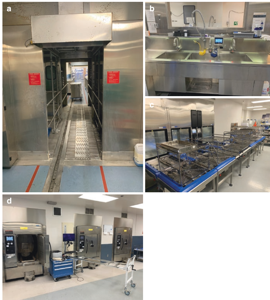
Fig. 10.8 Hospital sterile processing. There are several stages to sterile processing in hospitals and a significant amount of space and equipment is dedicated to processing. (a) Instrument cart cleaner. (b) Soak and sonic sinks. (c) Instrument washers on conveyor belt. (d) Steris sterilizers
