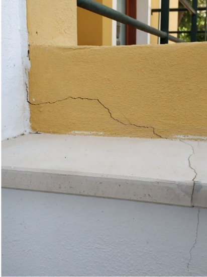
a) Joint displacement with implication to other elements of the contiguous dwelling.
