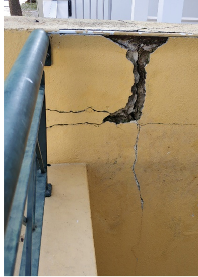
b) Cracking on the balcony wall.
