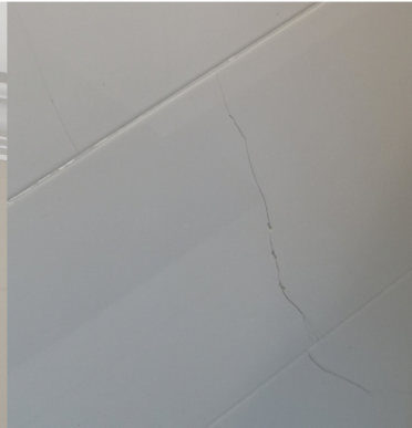
d) Tiles from the bathroom fractured.
