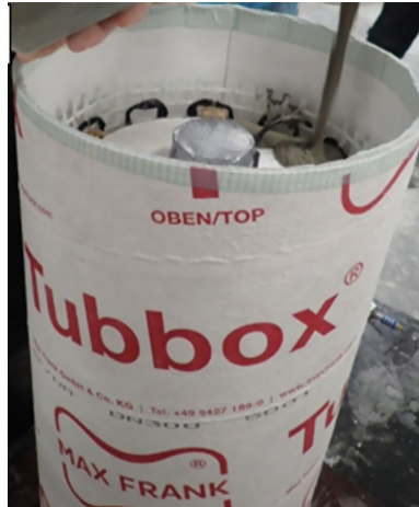
Fig. 15. Formwork variant for curved CCE: Tubbox formwork tube from Max Frank GmbH with polystyrene core.
