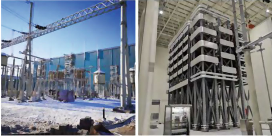
Fig. 13.31 535 kV DC circuit breaker in the Kangbanuoer converter station
