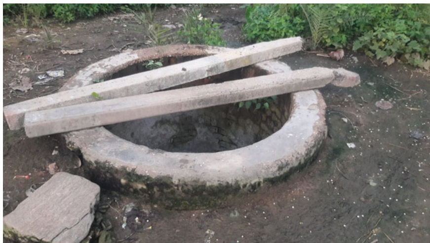
Fig. 16.3 Open Pat Kua structure at village Malthore of Belma GP in Purulia-2 block
