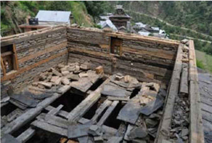
Fig. 24.37 Dry masonry with infill and lap-joined pieces at the corner. Source : “HV-Himalayan Vernacular,” Kath Kuni, Architecture and Visual Material Arts, 2018
