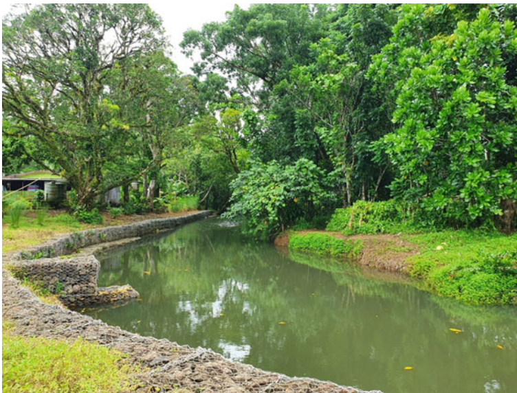
Fig. 7.5 Retaining wall at Nadaro Village. Source The corresponding author took a photograph
