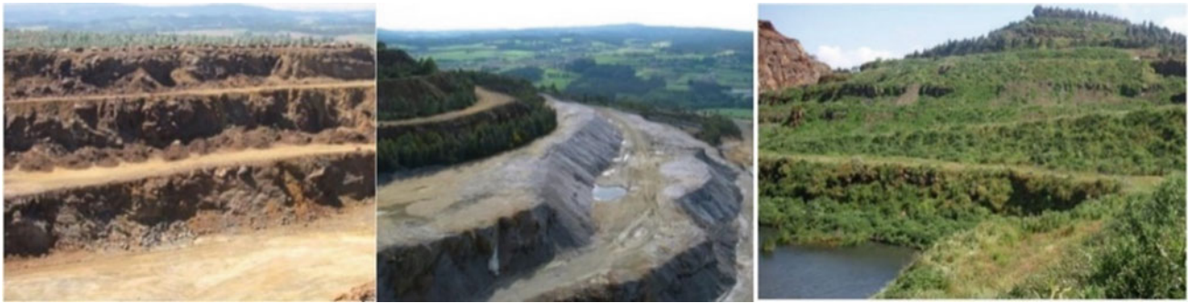
Fig. 2 Cu sulphide mine (Touro). Recovery of hyperacid cuttings with tailor-made Technosols (1998–2021). Surface runoff waters moved from pH < 3.5 to 7.0, recovering the whole trophic chain and
