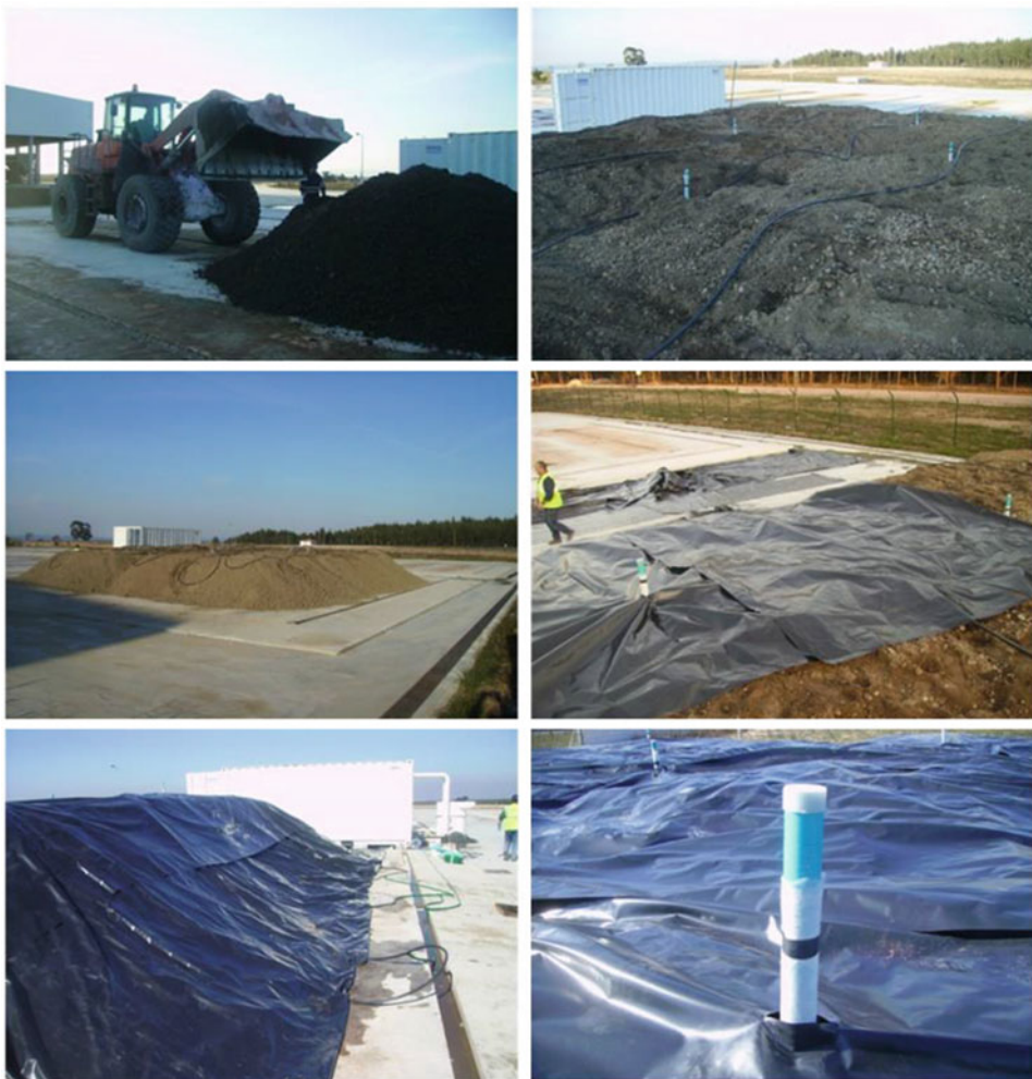
Fig. 1 Construction of a biopile (Photos kindly shared by CIRVER ECODEAL). From top to bottom and from left to right: 1—Spreading of the soil; 2—Installation of gas monitoring pipes watering system; 3—Biopile before impervious cover; 4—HDPE sheet extended over the biopile; 5—Watering system connection; 6—Gas monitoring pipe (detail)
