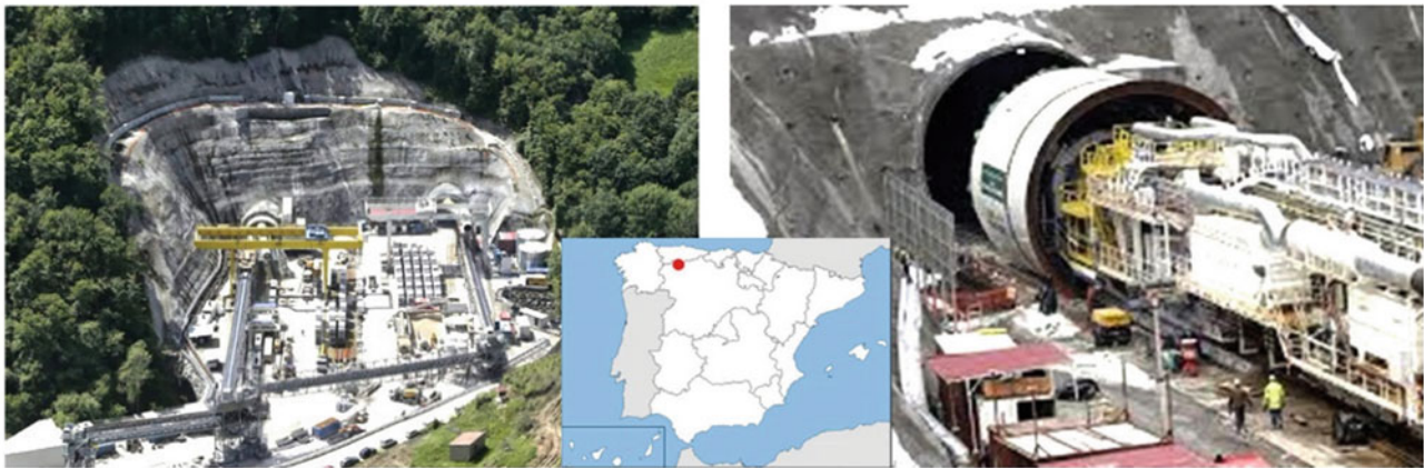
Fig. 1 Left: A general view of the Pajares Tunnels portal area. Right: Tunneling Boring Machine (TBM) used in the Pajares Tunnels. Photos ADIF, Administrator of Railway Infrastructures
