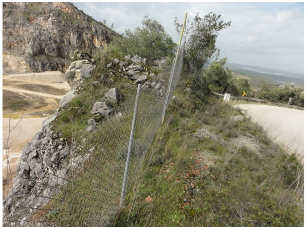
Fig. 1 Example from an insufficient safety distance of a high vertical quarry slope to a public road (photo: MQF)
