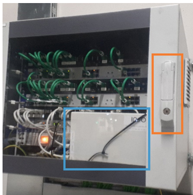
Fig. 6. COMSEC (in blue) on the locked airport switch cabinet (orange). (Color figure online)
