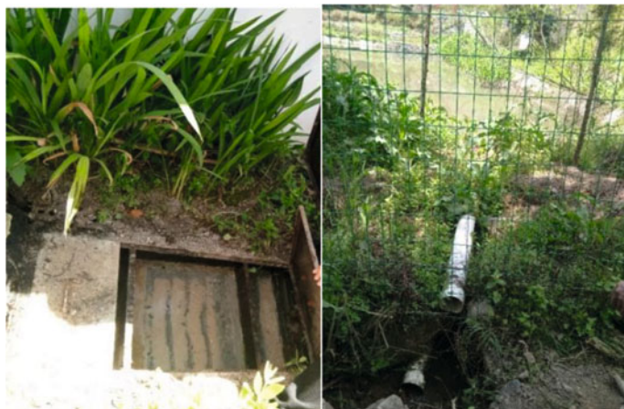
Fig. 59.2 Photo of oil separator and drain pipe
