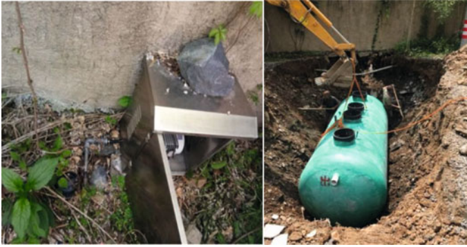
Fig. 59.3 Aeration pipe and micro power device of B&B Remote Mountain
