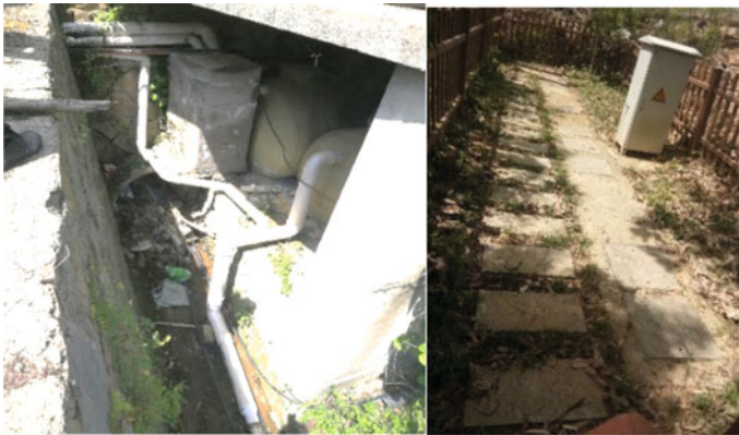
Fig. 59.1 Photo of sewage treatment facilities in Xiantan Village and Laoling New Village
