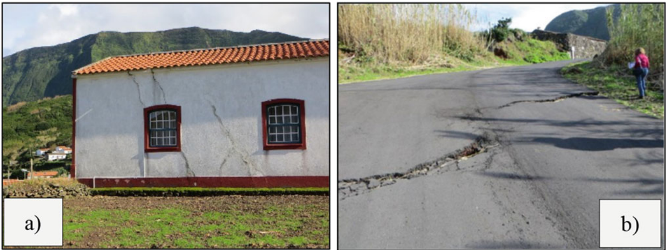
Fig. 3 Pathologies verified: a in housing; b streets
