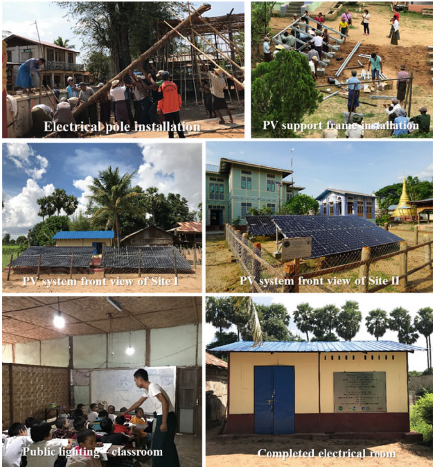
Fig. 3.2 Solar PV system and LED lights installation. Source Compiled by the author
