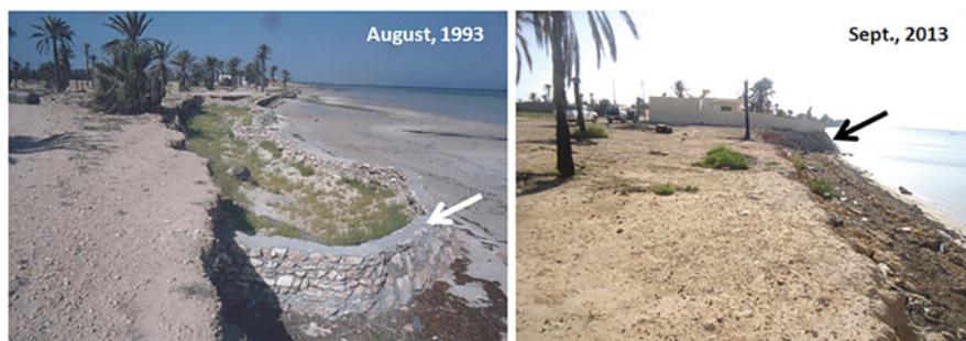
Fig. 12.18 One of the many illustrations of perseverance in reproducing the same mistakes in the Kerkena archipelago. Appearance of hard constructions in a clearly eroding coast. The arrows indicate the same low wall, originally (in 1993) created as a protective structure (photos, Ameur Oueslati)
