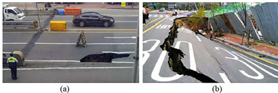
Fig. 1.5 Photographs of urban road sinkholes that were due to an underground void in the area: (a) Seokchon Station in Seoul, Korea (August 2014), and (b) Incheon, Korea (July 2014) (modified from Nam et al. 2018)
