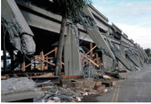
The upper level of Interstate 880 in Oakland, California, U.S.A., collapsed during the Loma Prieta earthquake (M=6.9) on October 17, 1989. 41 people were killed
