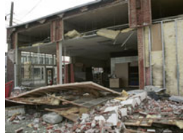
This business in Seattle was heavily damaged during the Nisqually, Wash., earthquake (M=6.8) on February 28, 2001. About 400 people were injured
