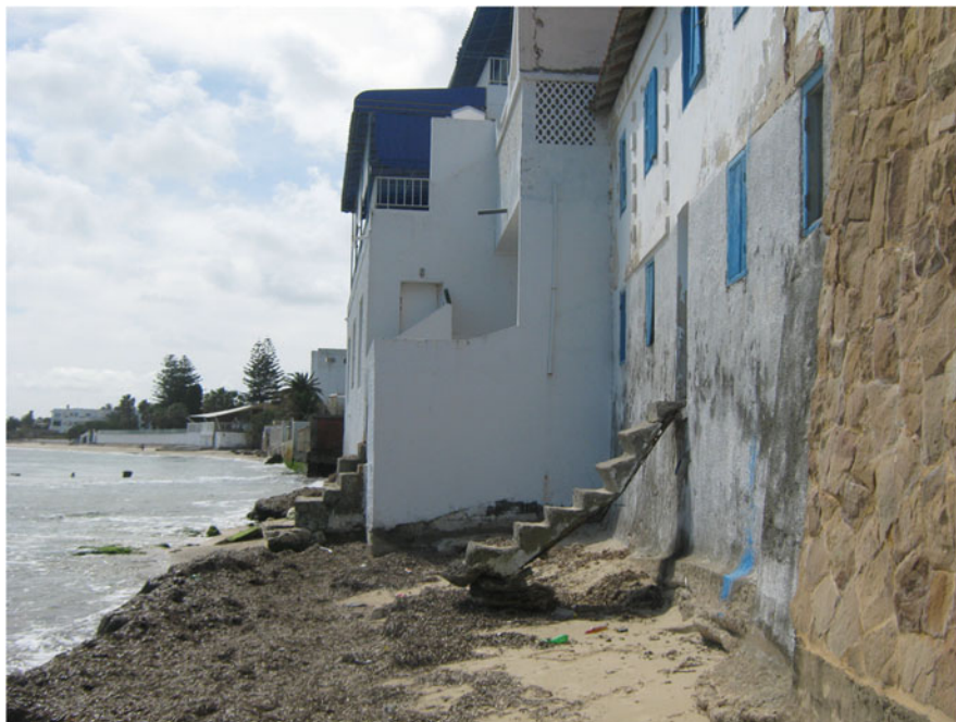
Fig. 12.11 The situation at the Corniche de Bizerte, in the vicinity of the Petit Mousse restaurant: the state of the stairs, witnesses of the important lowering of the surface of the beach (Photo, Ameur Oueslati, April 2010)
