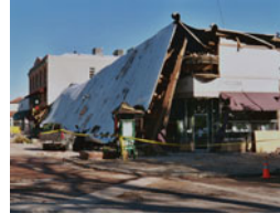
Building collapse in Paso Robles, Calif., during San Simeon, Calif., earthquake (M=6.5) on December 22, 2003. 2 people were killed
