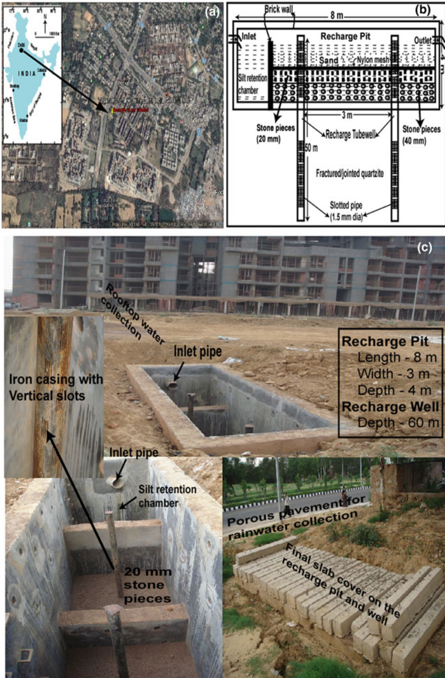
Fig. 19.2 Construction of recharge pit and tube well to harvest rooftop rainwater in the Vasant Kunj urban housing colony, New Delhi. a Location map of the study, b schematic recharge pit and well diagram, c photos of the recharge pit and tube well construction site (photo: May 2012)
