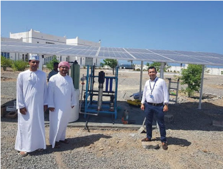
Fig. 3 A pilot photovoltaics (PV)-RO unit installed at the Middle East Desalination Research Center ( 1.3 \text{ m}^3/\text{h} ). Project carried out by researchers from SQU and MEDRC
